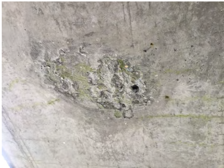
Spalling on concrete slab 3
